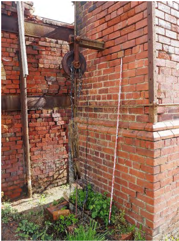
Figure 22 Pulley for operating the flue damper (G. Vines 10/5/2023)
