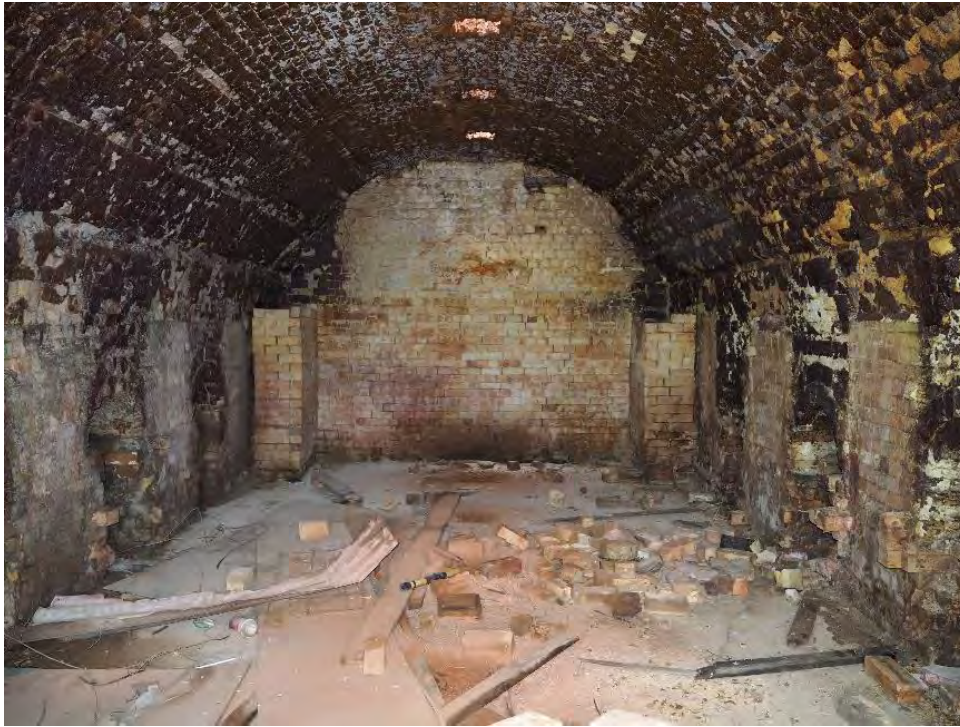
Figure 15 Looking into rear of kiln (towards east) showing surviving fire hole baffles at far end (G. Vines 10/5/2023)
