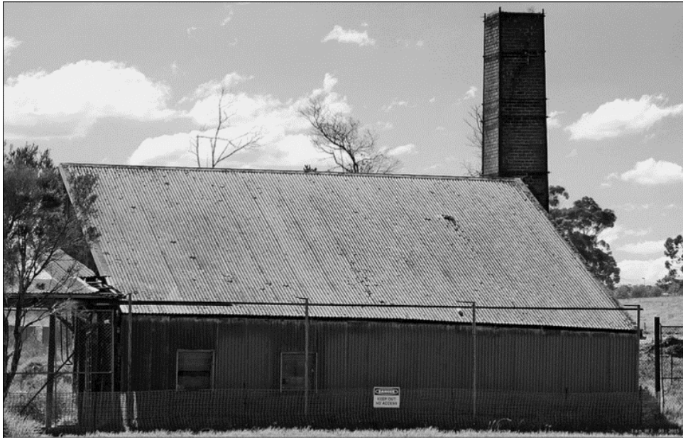
Figure 10 Hicks Pottery prior to collapse of roof (photo Graeme Butler)
