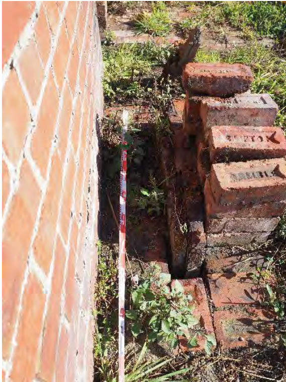
Figure 20 Flue damper on north side of chimney (G. Vines 10/5/2023)
