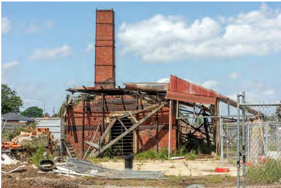
Figure 11 Hicks Pottery after much of the roof blew off in November 2018 32
