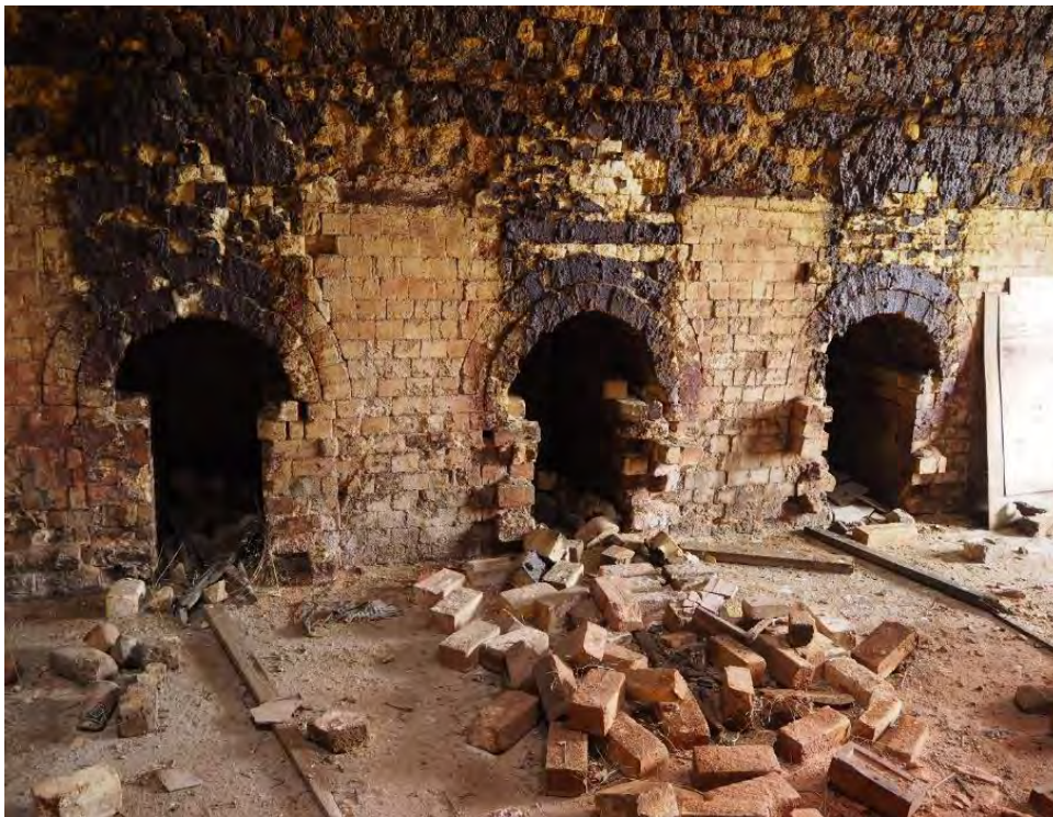
Figure 14 Interior of kiln showing flaking surface of fire glazed brickwork and remains of Firehole baffles (G. Vines 10/5/2023)
