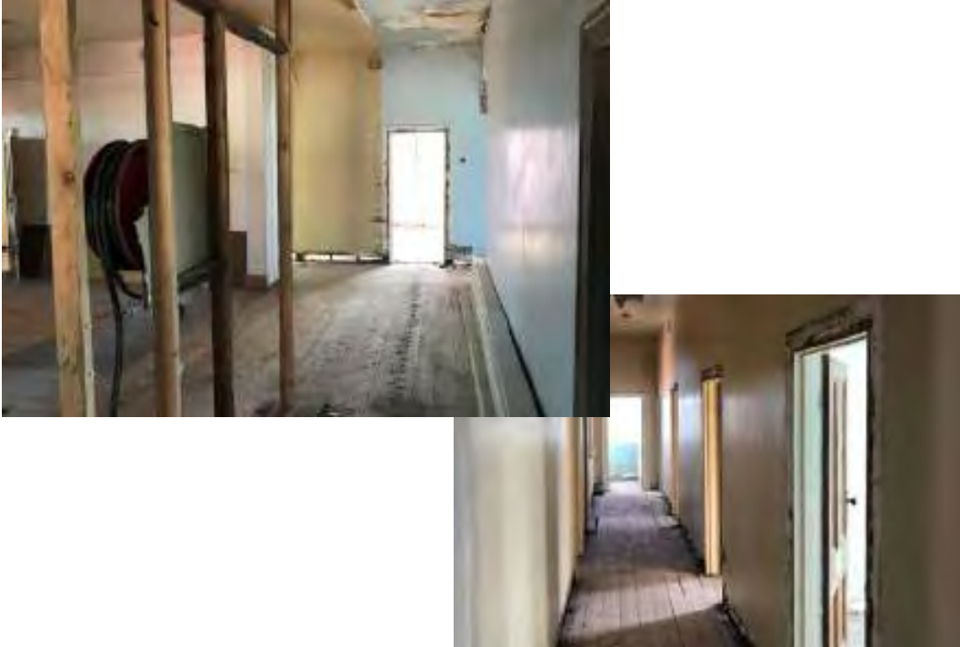
Image 6| Upstairs is presently derelict and unused
