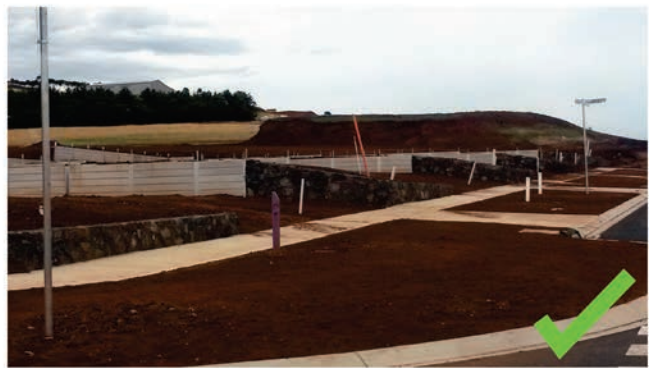
Where pre-development slope is less than 10%, consider how pre-benching lots and including retaining walls could manage site cut and fill and limit conflict between lots
