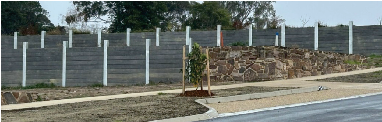
Figure 26 - Example of rock retaining wall along the property frontage and initial front setback, with concrete sleeper retaining wall behind the building line
