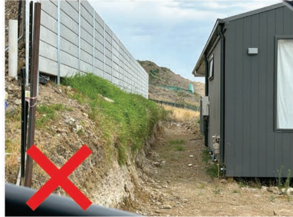
Ensure side boundary retaining is coordinated along lot boundaries to avoid excessive cut and high retaining walls
