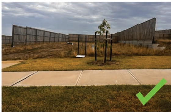
Subdivider has pre-benched and included retaining walls and fences on lots to ensure suitable buildable pads for dwellings
