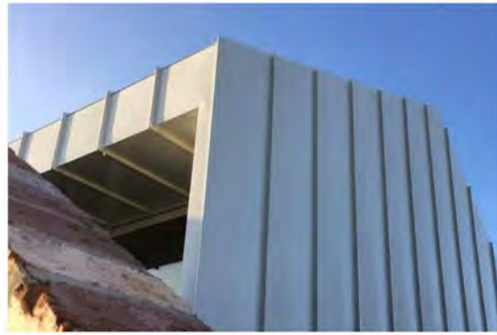
CLM-01 METAL CLADDING: Vertical - 'Standing Seam' Cladding Profile or similar - Powdercoated Colorbond Steel 'Surfmist' or similar
