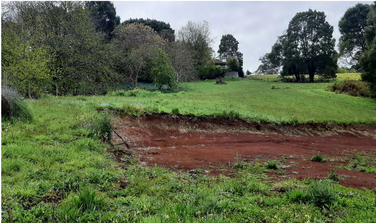
IMAGE 10 - Location of Building Envelope with existing site cut. View to the north (rear) of the site.
