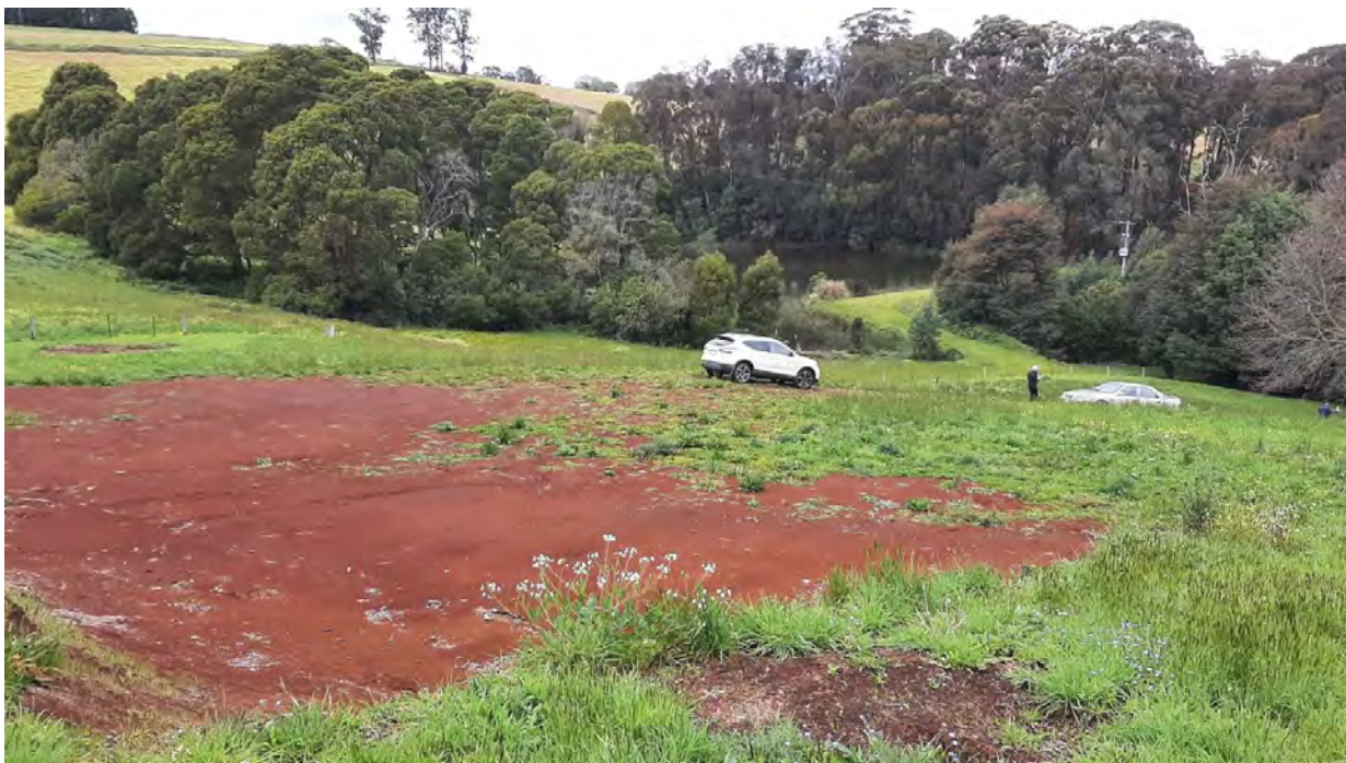
IMAGE 9 - Location of Building Envelope with existing site cut. View to the south east of the site.
