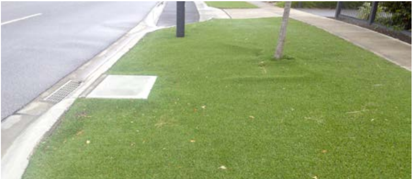
Synthetic turf not installed correctly – lumps, dips, not flat.
